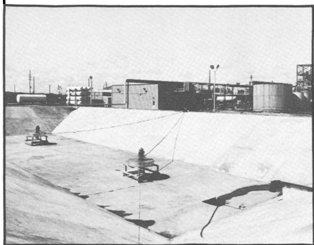
Part of the two part waste treatment system at the Painesville, Ohio facility of Glyco Chemicals, Inc. Shown in the skimming basin used for fat recovery where wastes are aerated (two aerators are shown in bottom of basin.) Wastewater is combined with boiler blowdown and sanitary wastes in final collection sump, then pumped to equalization basin and subsequently to a regional treatment system.
